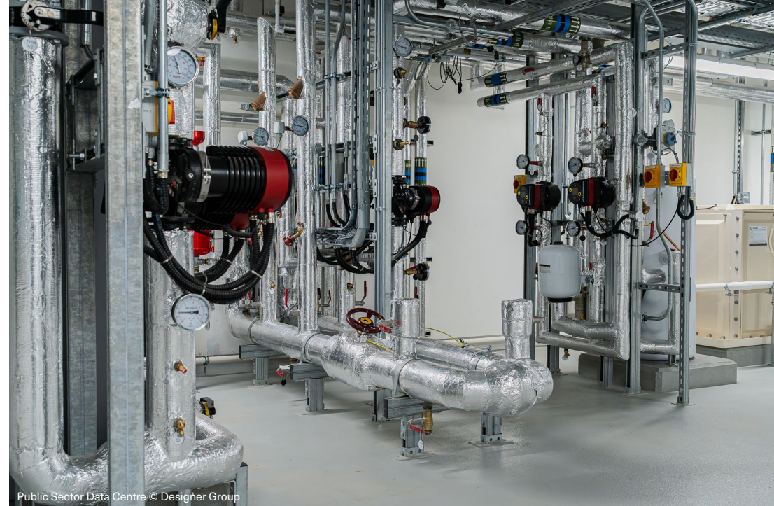
Public Sector Data Centre © Designer Group
